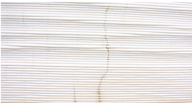
Example of hairline cracks in 3DPG
